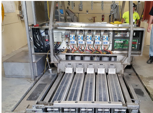
Photo: Bucklin Point UV Disinfection System
