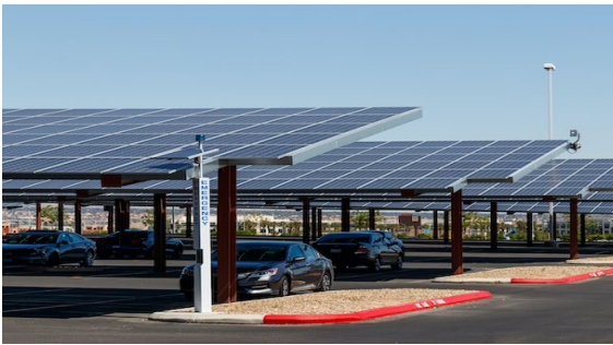
Photo: Solar Carport
