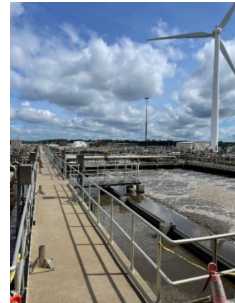
Field's Point Aeration Tank
