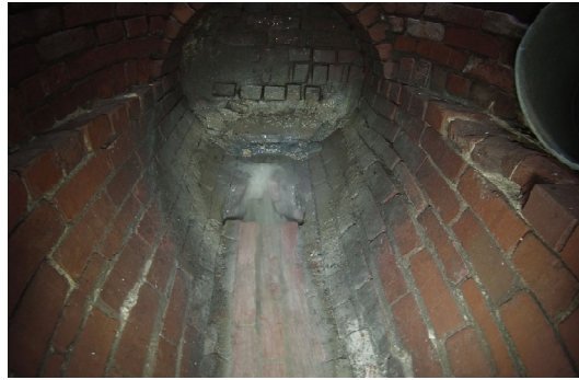
Photo: OF 056 Regulator on Vandewater Street
