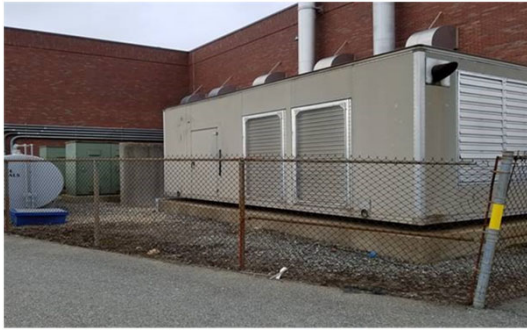
Photo: Field's Point Screw and Blower Generator
