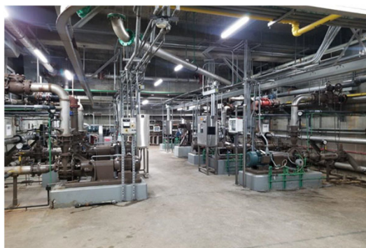
Photo: Primary Sludge Pump Station
