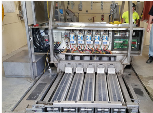
Photo: Bucklin Point UV Disinfection System
