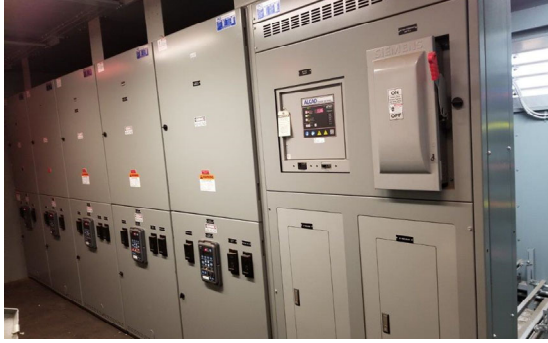
Photo: Field's Point Electrical Facility
