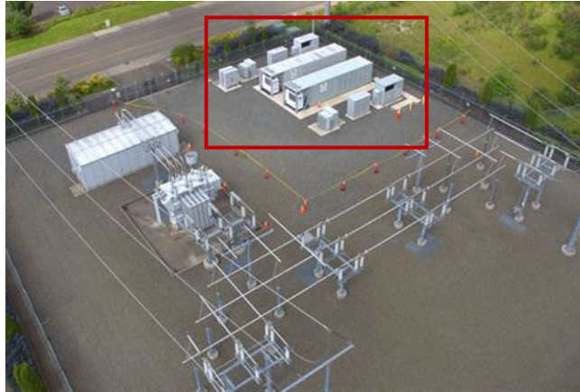
Snohomish Public Utility District (WA), Wind Power Monthly
