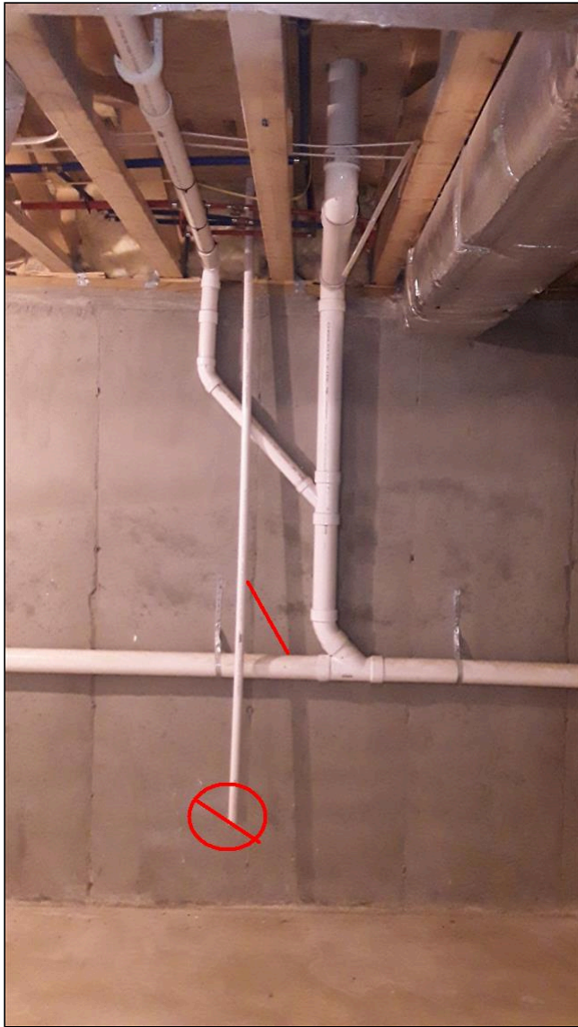
5.0 Item 3(Picture) (4) Trip waste needs repair or replace as needed
