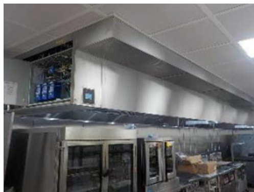
CaptiveAire hood – Main kitchen
