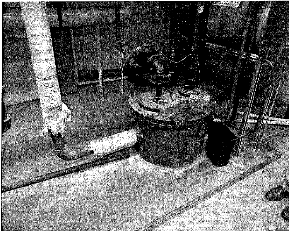
Photo B-24: Boiler Blowdown
