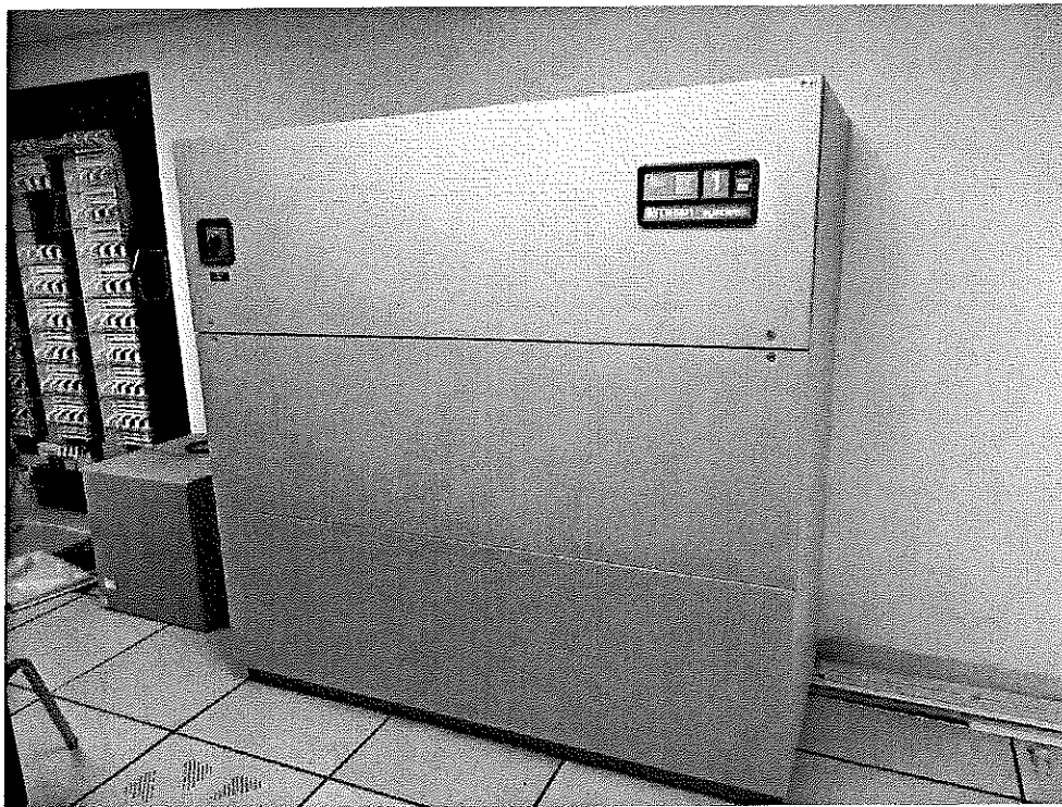
Photo B-42: Liebert Air Conditioning Unit
