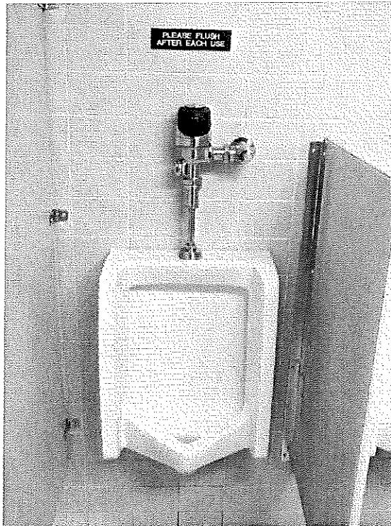
Photo B-5: Urinal (Typical)
