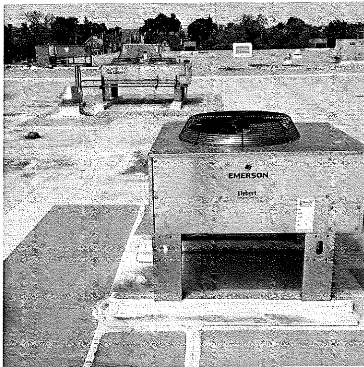
Photo B-44: CRAC Rooftop Condensers (Typical)
