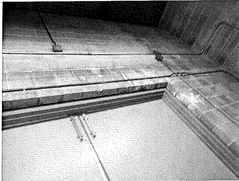
Photo A-3: Generator house concrete masonry bearing/shear wall with efflorescence visible
