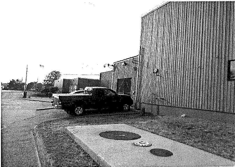
Photo A-10: Minor damaged to façade at adjacent parking area on southern wall
