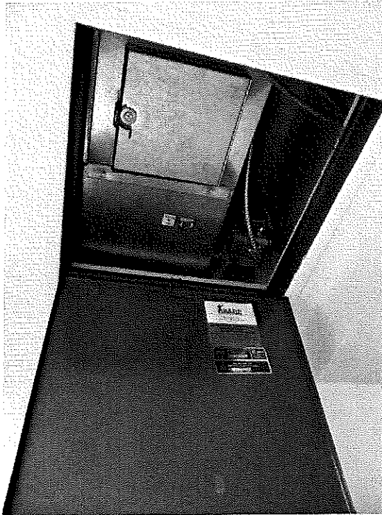
Photo B-52: Ductwork Fire Damper (Typical)
