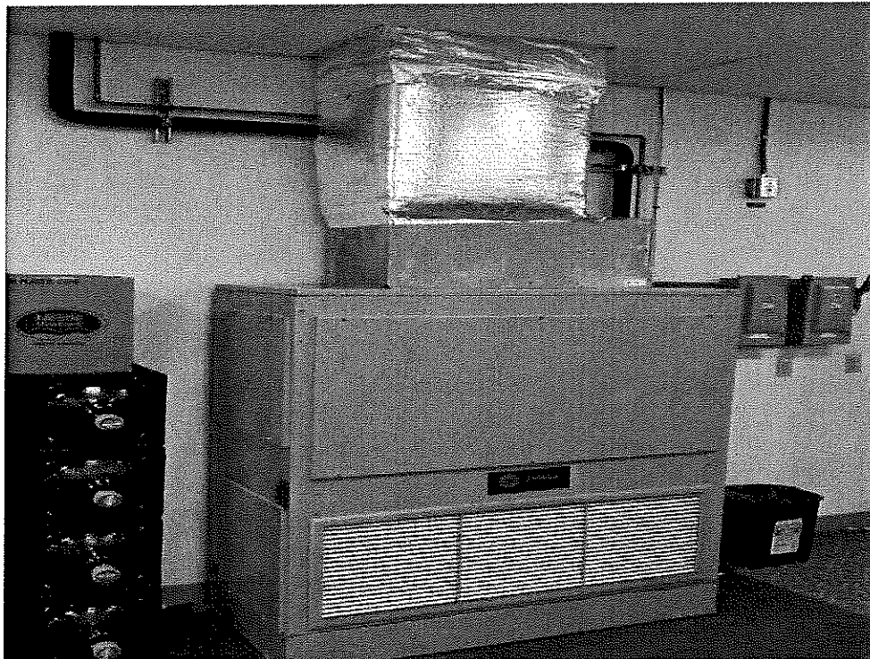
Photo B-34: Indoor Trane Air Handling Unit with Electric Heater (Typical)
