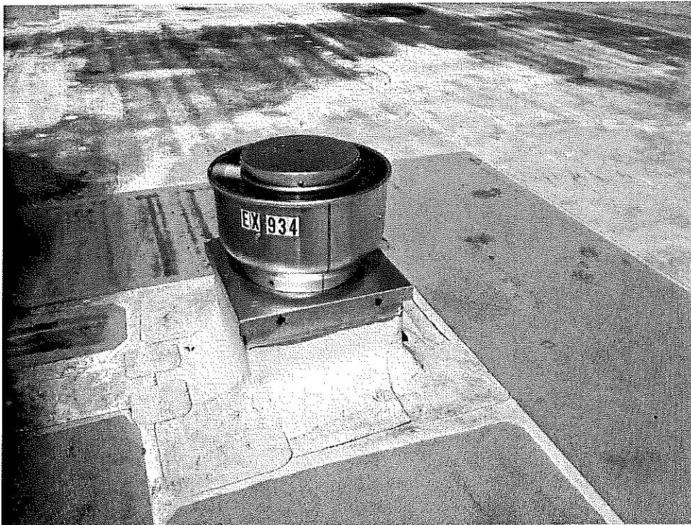
Photo B-16: Kitchen Ventilation Hood Exhaust
