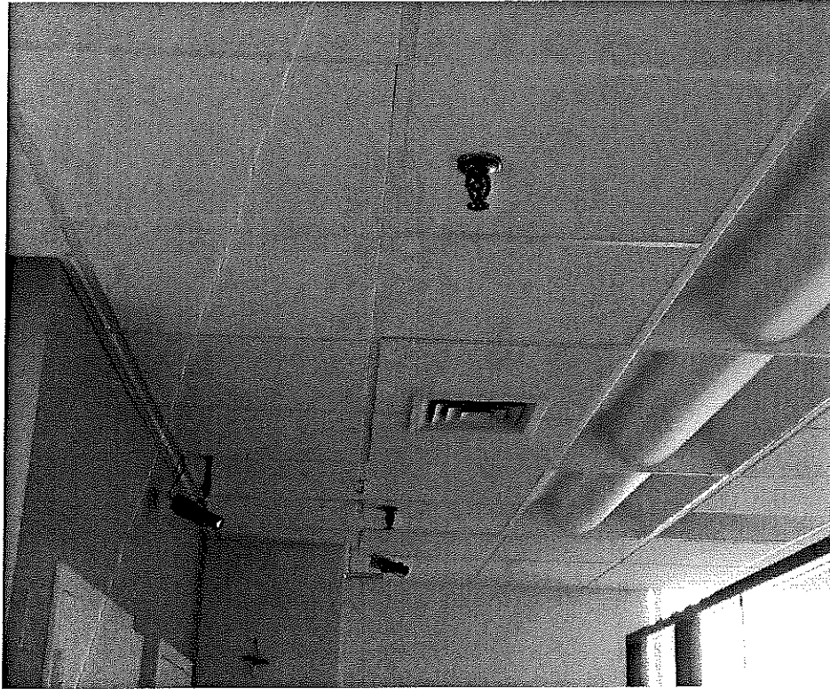
Photo B-50: Sprinkler and Diffuser (Typical)
