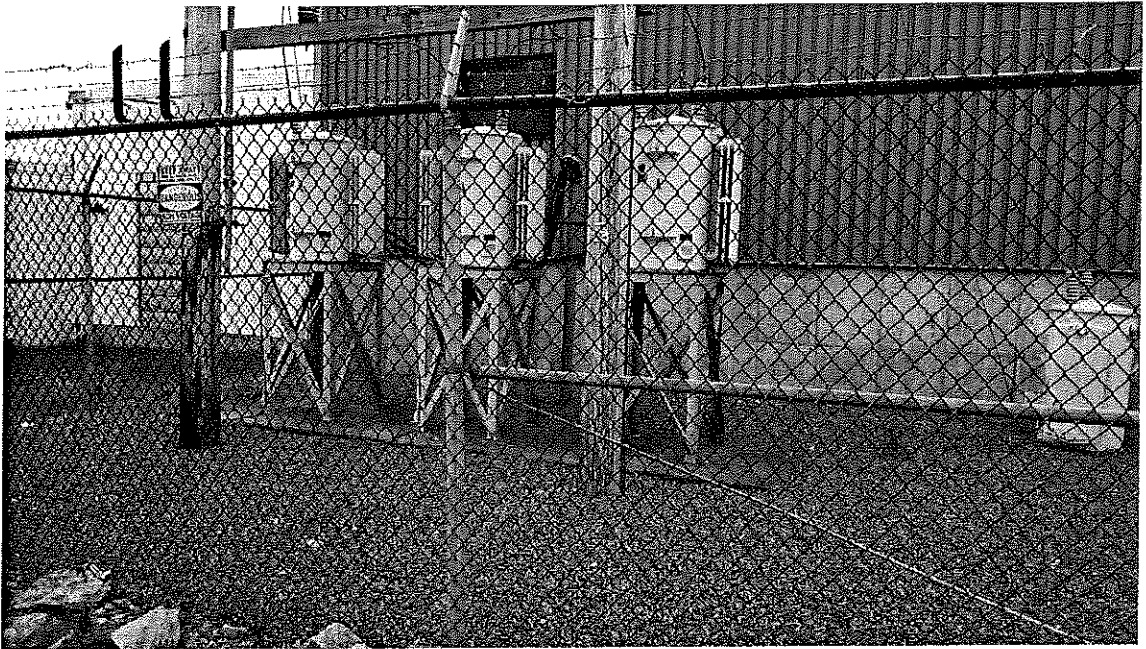
D-11: Transformer banks- North end of property (looking south)
