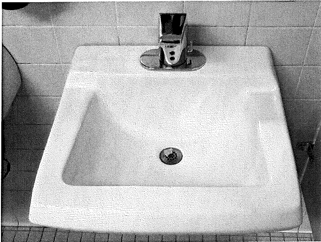
Photo B-2: Sink (Typical)
