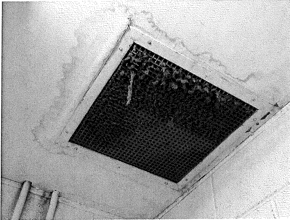
Photo B-27: Dirty Exhaust Grille
