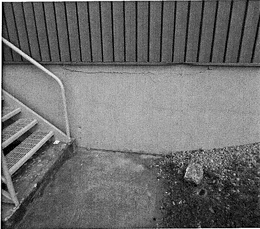
Photo A-1: Foundation crack at westernmost loading dock along north wall
