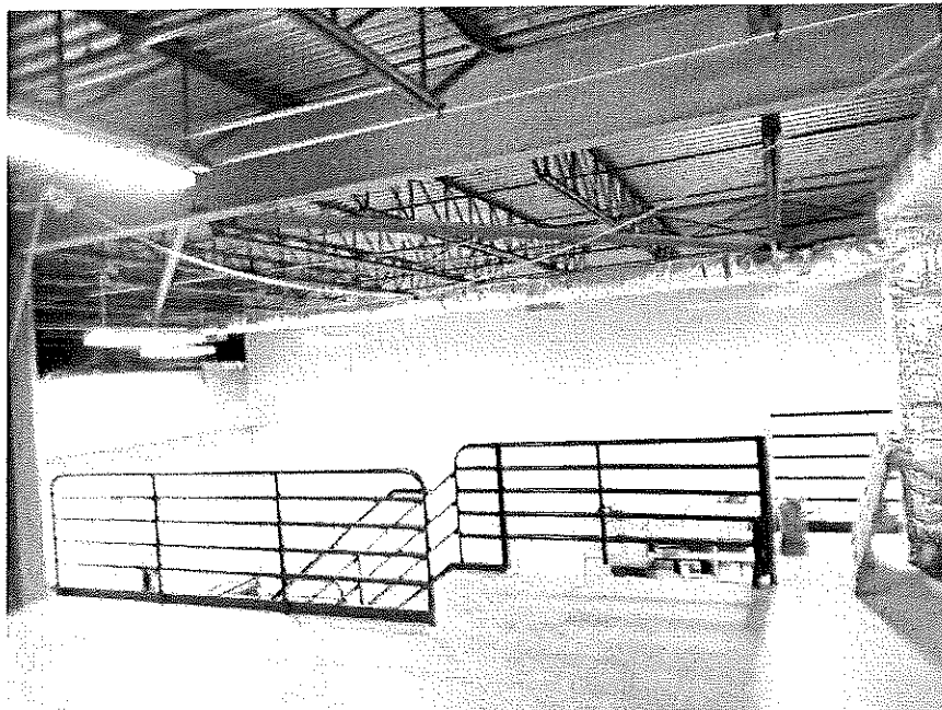
Photo A-2: Storage area located within main building exhibiting typical roof framing
