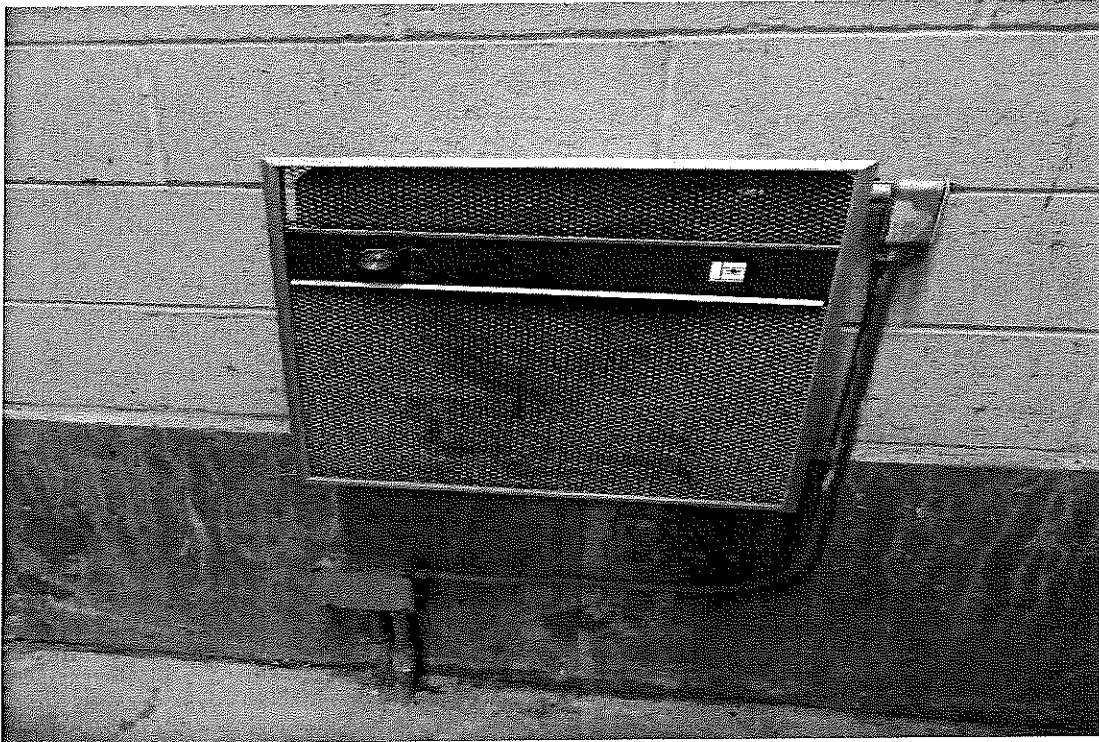
Photo B-29: Electric Cabinet Unit Heater
