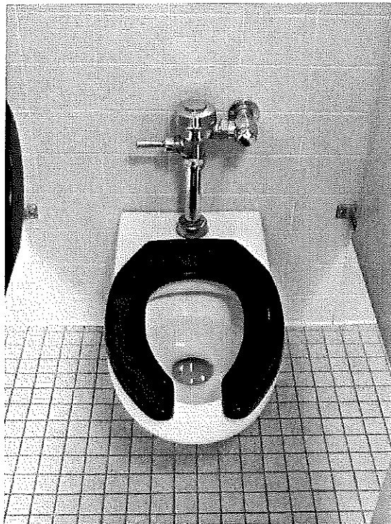
Photo B-6: Tankless Toilet (Typical)
