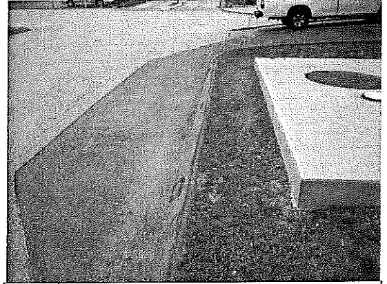
Photo #10: Area of former leaking underground storage tank
