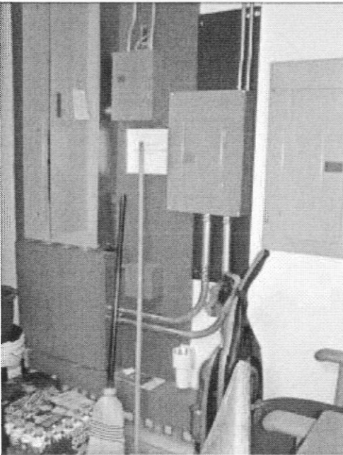
Cranston Electrical Panels
