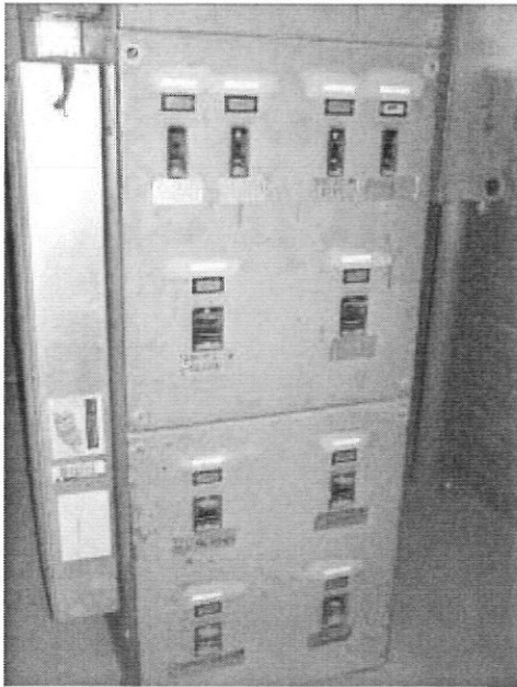
Providence Electrical Gear
