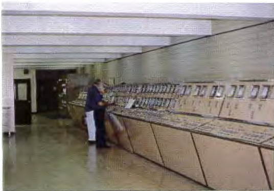
Old analog Central Control Board at treatment plant
