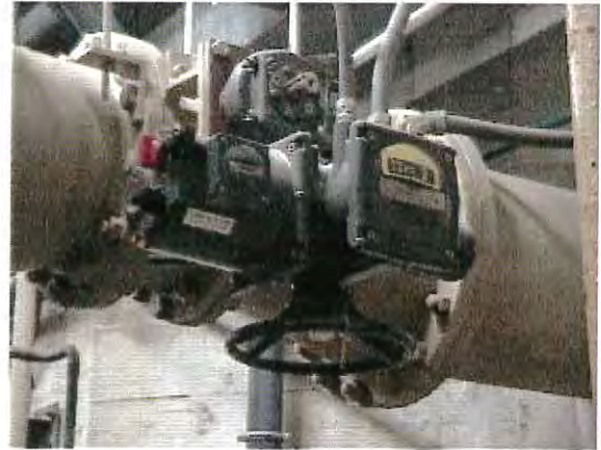
Typical new effluent valve actuator at treatment plant providing precise plant effluent control
