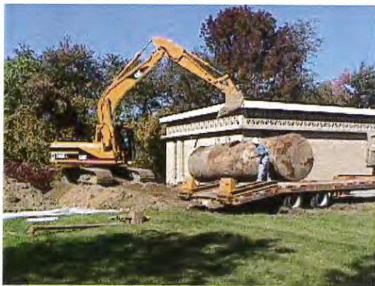
Removal of old underground fuel storage tank at the Western Cranston Pumping Station
