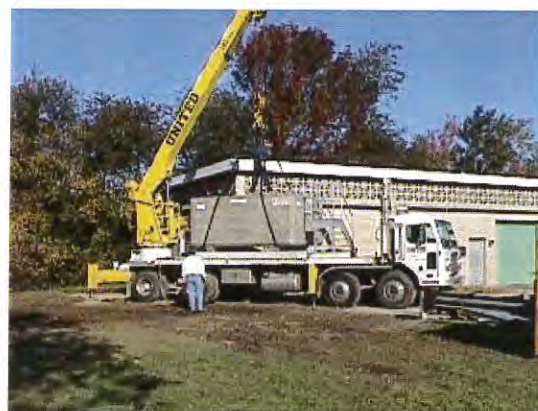
Delivery of new above ground fuel storage tank at the Western Cranston Pumping Station
