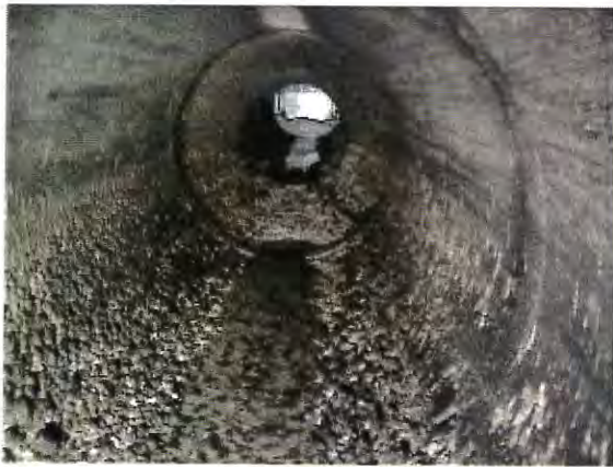
Concrete corrosion damage to the lower half of the effluent conduit
