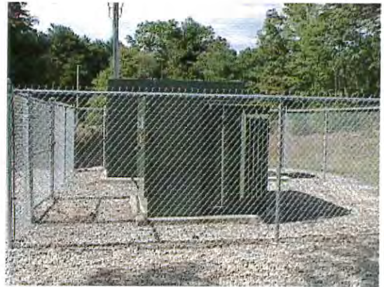
New 23,000 / 2,300 transformer and switchgear replacing obsolete electrical feed system to the treatment plant
