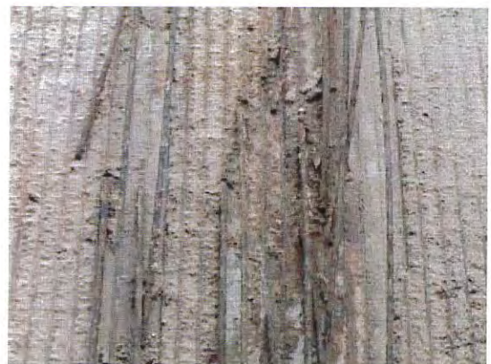
Close-up of failed pre-stressed wires of the 102" Aqueduct
