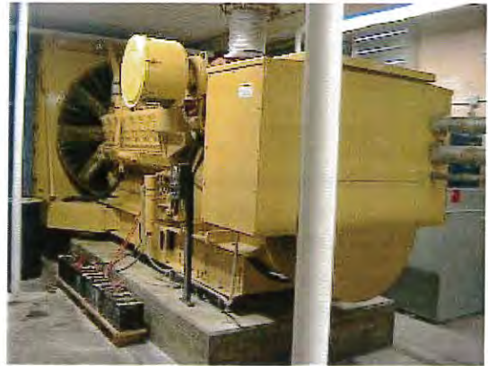
New Raw Water Booster Pump Station generator for backup power to treatment plant
