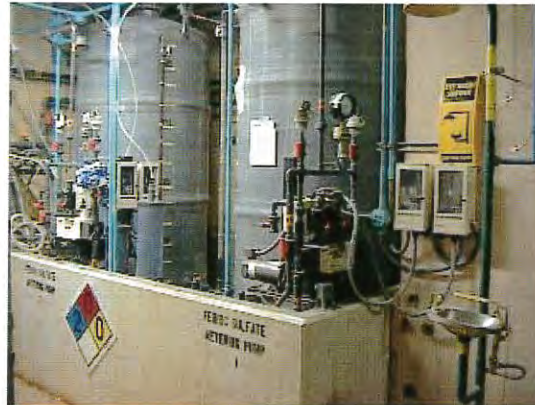
New sulfate feeder equipment and day tanks for liquid ferric sulfate coagulant injection
