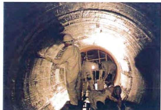
Crew applying Carbon Fiber Lining to interior of deteriorated section of 102" Aqueduct
