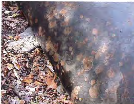
Exterior corrosion of 48" steel transmission main prior to rehabilitation
