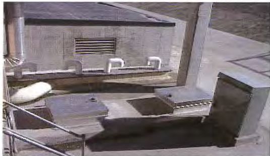
New Access Hatches and instrumentation panel installed over the opening of the venturi meters
