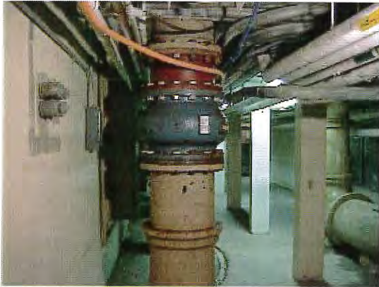
One of two new 18 inch check valves on suction lines to wash water pumps
