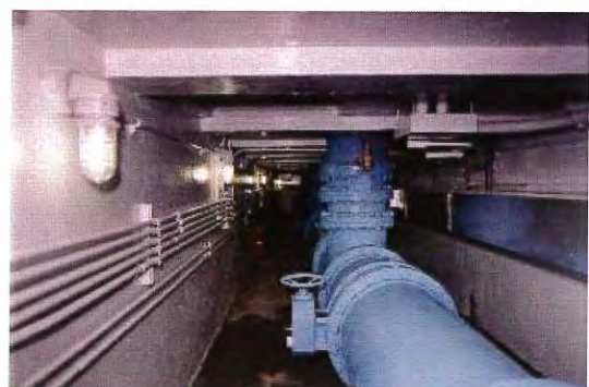
Neutaconkanut Pump Station piping after rehabilitation
