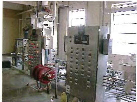
Two of four new lime feeders installed at treatment plant
