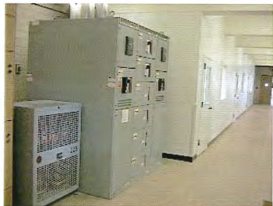
New 480 volt transformer and motor control center at treatment plant
