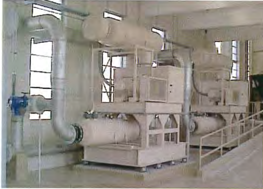
New air blower system at treatment plant for air scour backwashing of filters
