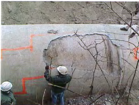
Exposing deteriorated section of 102" Aqueduct discovered through interior echo testing
