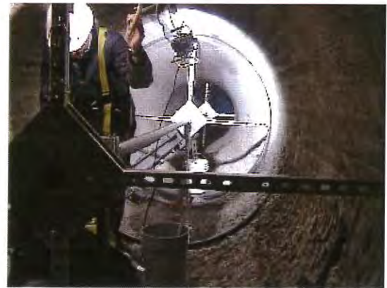
Concrete reconstruction and installation of new instrumentation in treatment plant's 72" x 42" effluent venturi meter
