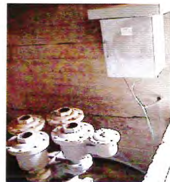
Electrical rectifier to provide cathodic protection to the twin 60 inch mains feeding raw water to the treatment plant
