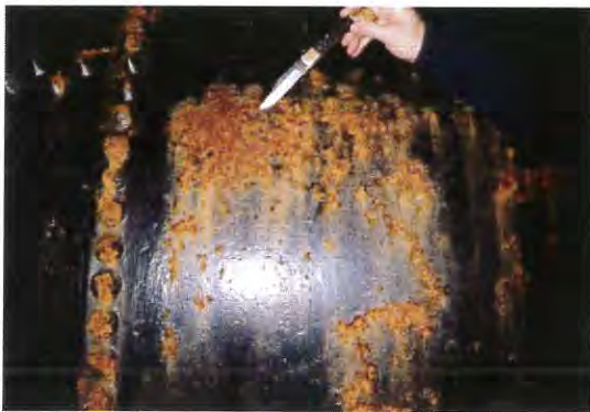
Corrosion on 60 inch main prior to rehabilitation
