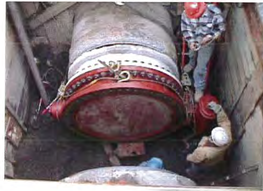
Installation of a new 60" butterfly valve to replace a defective valve at Budlong Road
