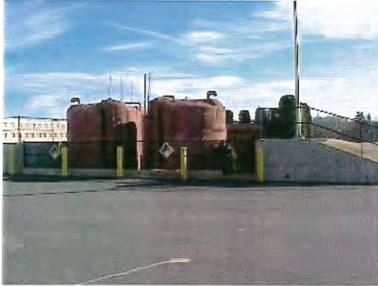
New liquid ferric sulfate storage tanks for new chemical feed system
