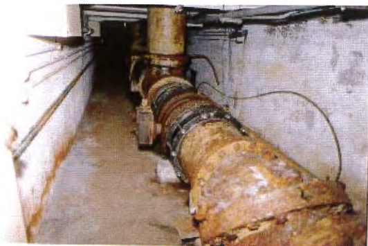
Neutaconkanut Pump Station piping before rehabilitation
