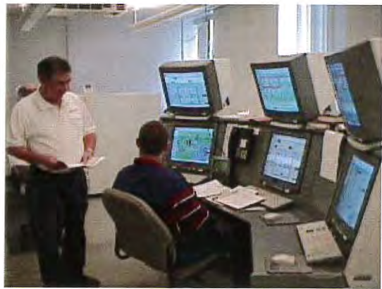
New state-of-the-art computerized Central Control System
