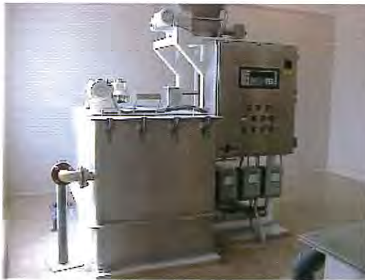
New fluoride feed equipment at treatment plant
