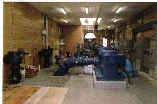
Bath Street Pump Station after upgrade
