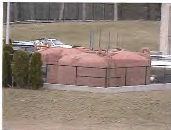
Ferric Storage Tanks
