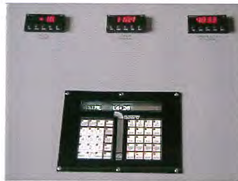
New electrical control system for Western Cranston Pump Station
