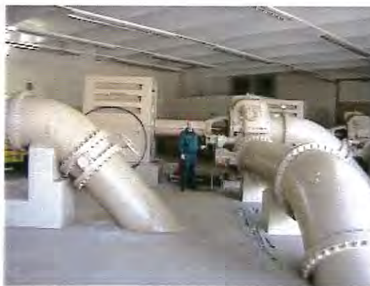
Existing Raw Water Booster pumps and valves
