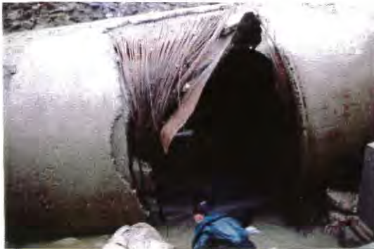
Rupture of the 102" Aqueduct – November 17, 1996
