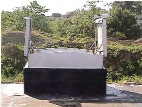
Installation of new access hatch into the 43 million gallon Aqueduct Distribution Reservoir
