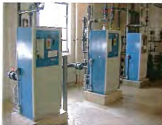
New automated chlorine feeders at treatment plant
