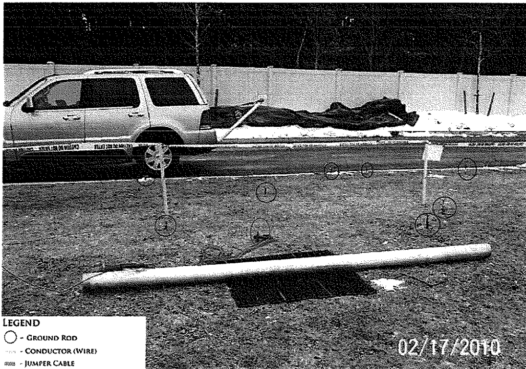
Figure 3 Photo from p 16 of L3 [Narda] test report, showing an array of added electrodes and ground rods added which boost the E-field signal from the substitute structure (Legend added)
