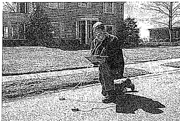
Photo Caption -Shawn Menear, a graduate student in Technology Education at West Virginia University, uses geophones to listen for water main leaks. Similar to a doctor or nurse's stethoscope, geophones are an inexpensive leak detection device used by water utilities. Photo by Eric Merrill.
