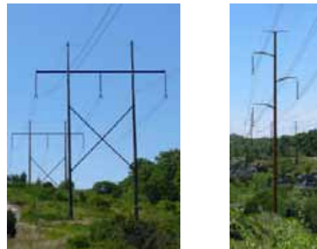
Figure 2-8. Photos of a wood “H” frame and a steel “monopole” designs.
