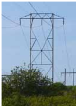
Steel Lattice Tower
